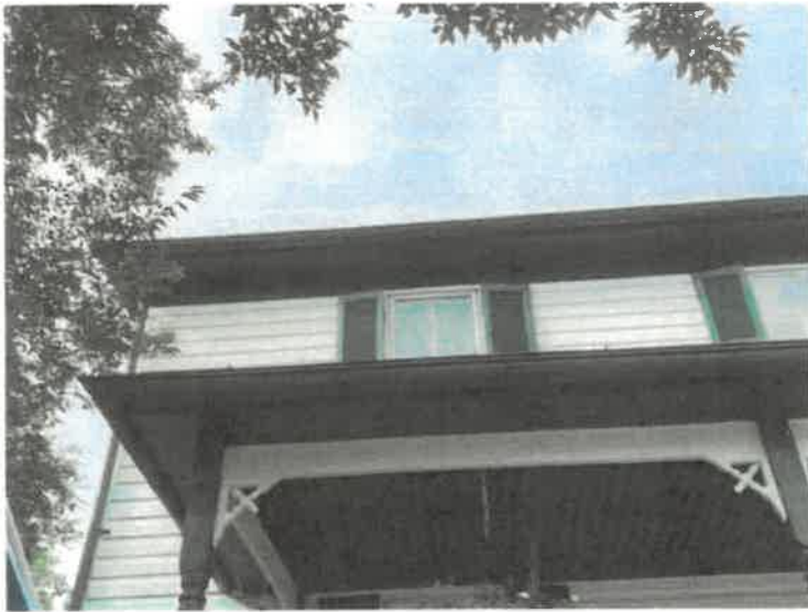
What the front gutters look like from the ground. These are 4"
