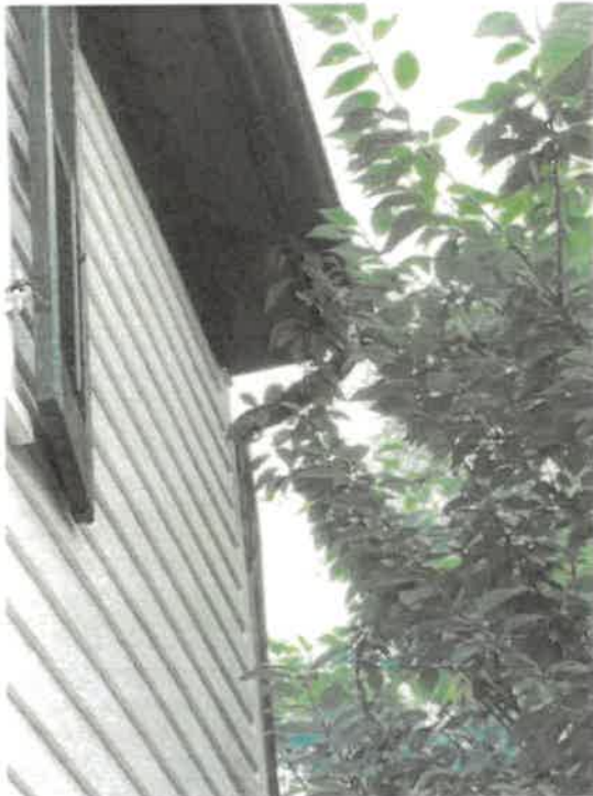
This is the downspout and underside of the existing 6" gutter on the north facing side of the roof to compare how it looks from the ground, compared to the 4" gutter in the front.
