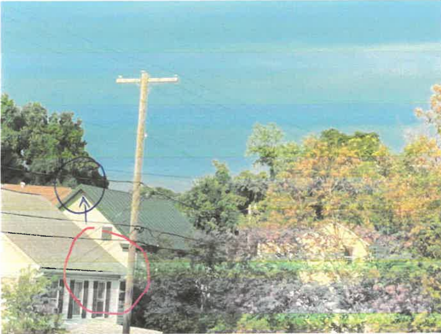
This shows the relatively steep angle of my metal roof. This is the south-facing side.
